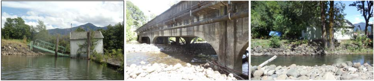
Figure 4.4-3 Potential Restoration Opportunities, Rock Creek Reach 1 Dilapidated structures and City-owned facilities present opportunities for restoration.
