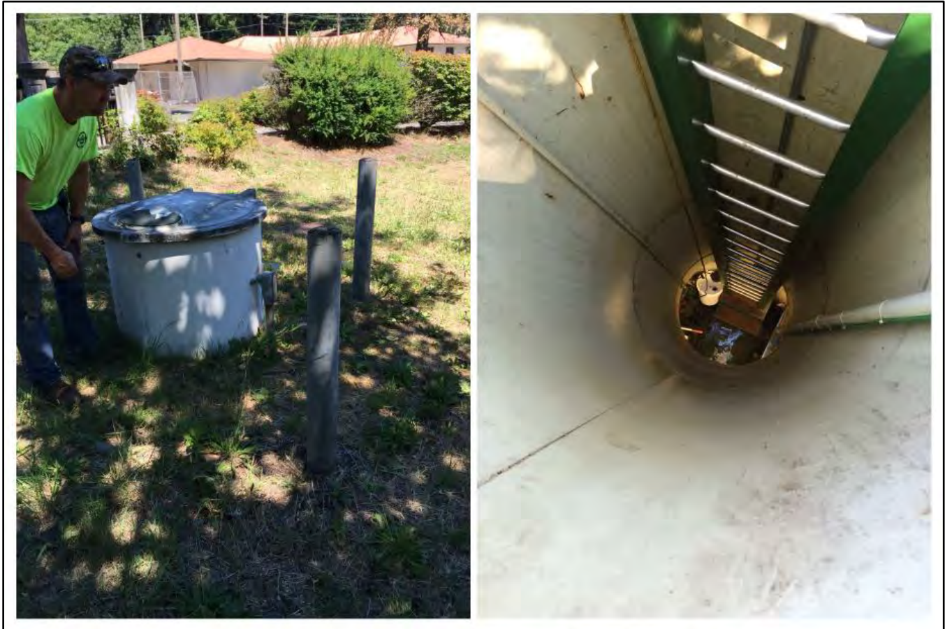
Figure 3-4. Rock Creek Pump Station Photos
