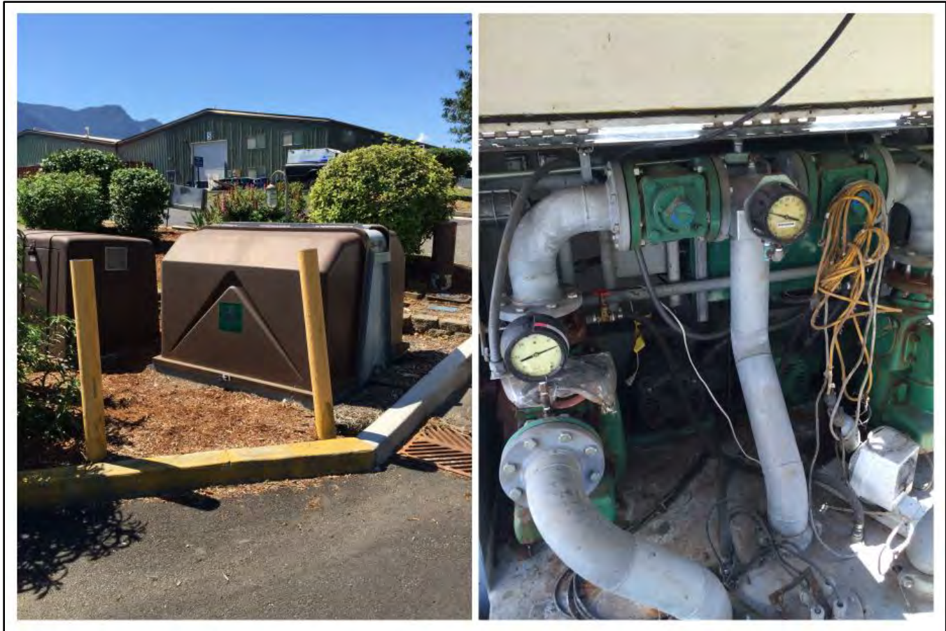
Figure 3-6. Kanaka Pump Station Photos
