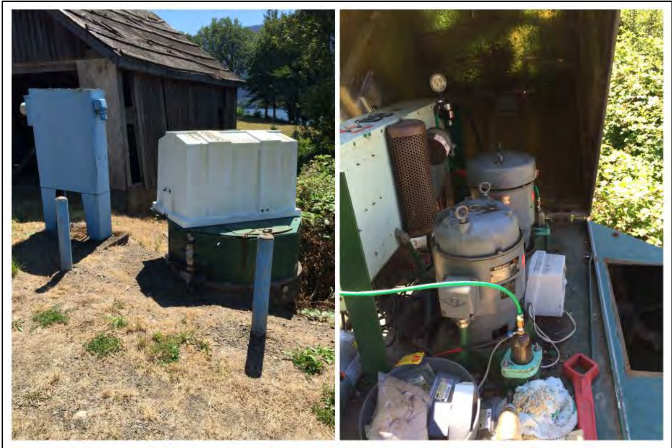
Figure 3-7. Cascade Pump Station Photos
