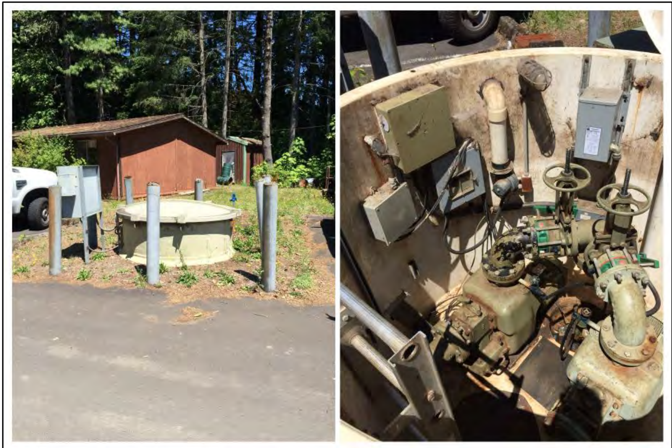
Figure 3-5. Fairgrounds Pump Station Photos
