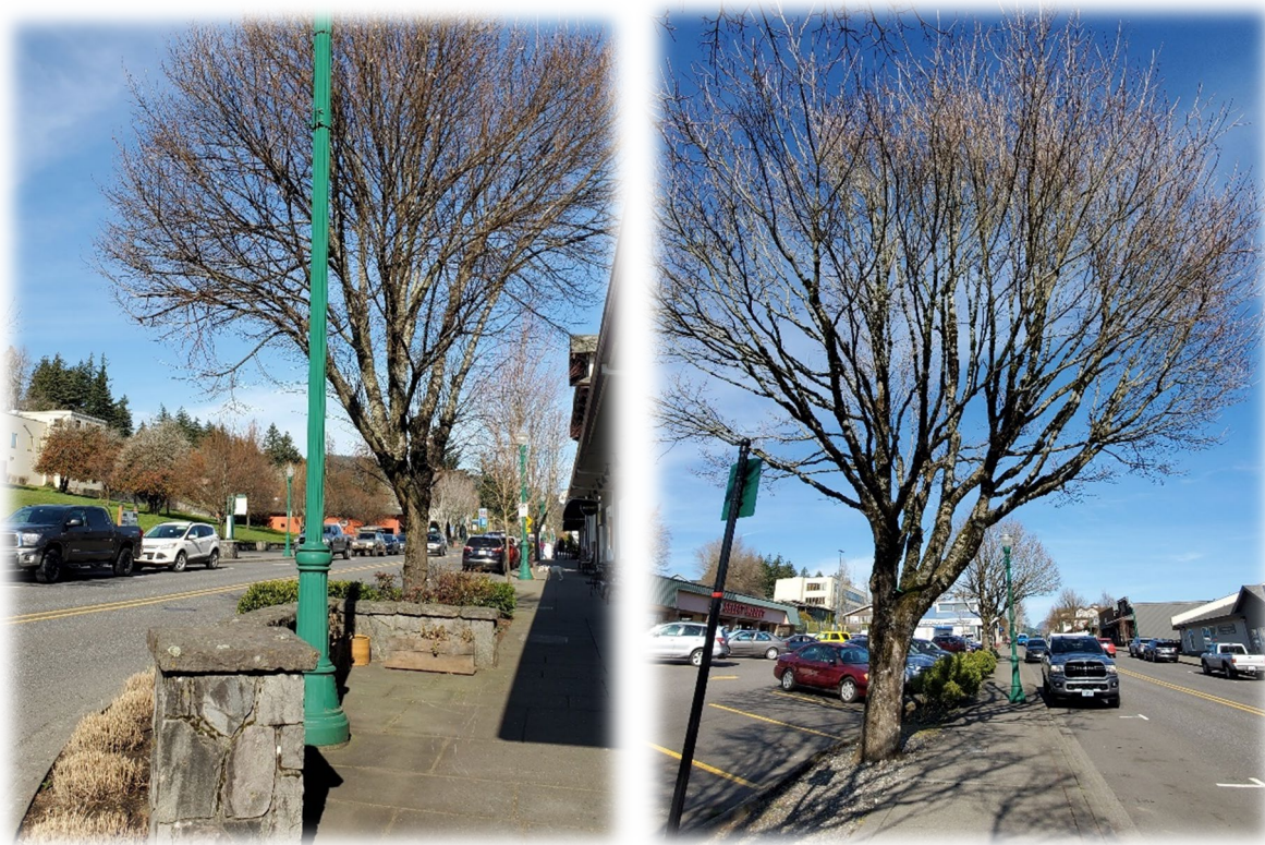
Photo36, 37. Tree #98 and 114 are mature and cannot be easily pruned for correction. Both canopies can be cabled to prevent future snow, ice and storm damage.
