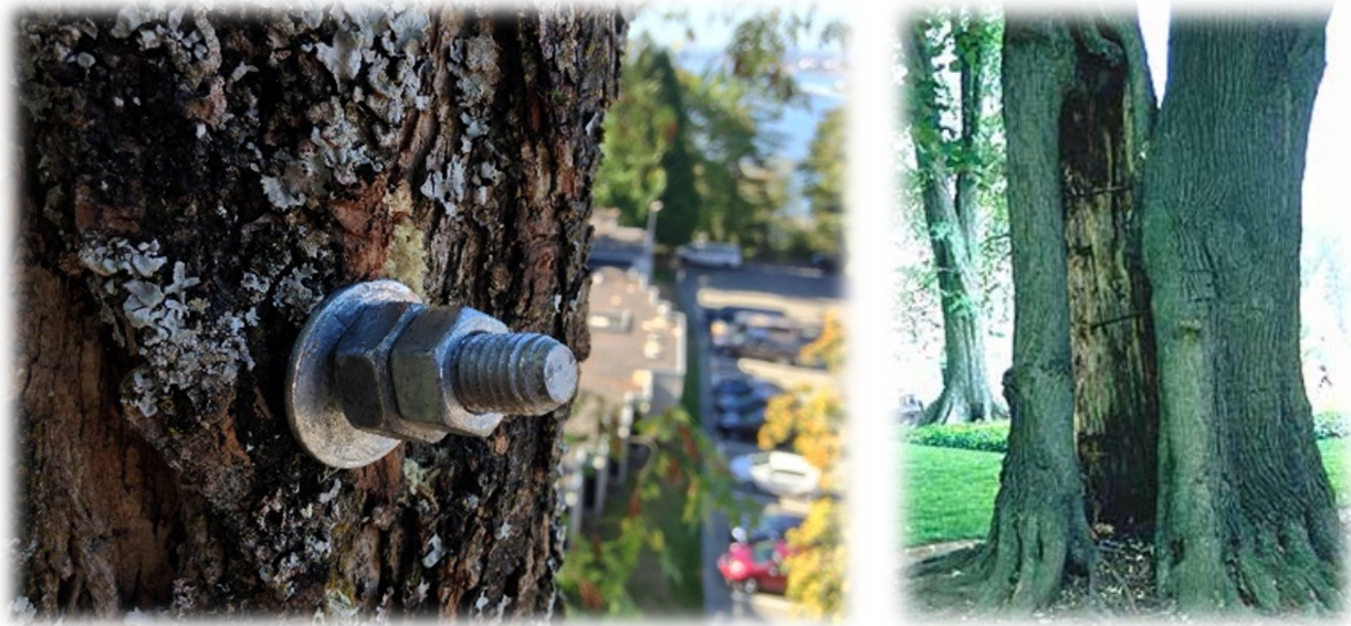
Photo 32, 33. Bracing the trunk of this tree will decrease the risk of failure. These braces should be supplemented with cables higher in the canopy to reduce movement. Illustrations, PowerPoints or photos by Edward F. Gilman, Professor, Environmental Horticulture Department, IFAS, University of Florida." http://hort.ufl.edu/woody
