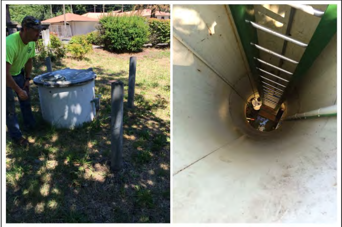
Figure 3-4. Rock Creek Pump Station Photos
